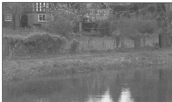
Damage done to a wall by the blast of bomb number 8 can still be seen today
